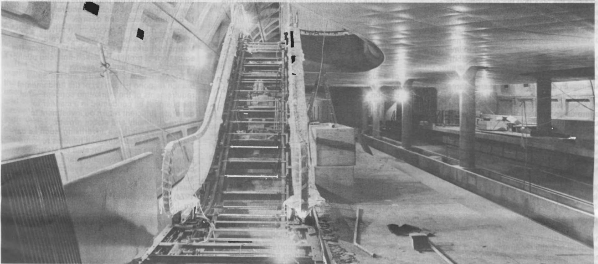
ESCALATOR UNDER CONSTRUCTION —Metro escalators will feature bronze cladding. Escalators between mezzanines and platforms will have glass sides for easy visibility and passenger safety. Metro designers many years ago decided to simplify the architecture to provide long sightlines and a minimum of obstructions to discourage crime. This escalator is at Judiciary Square station.
