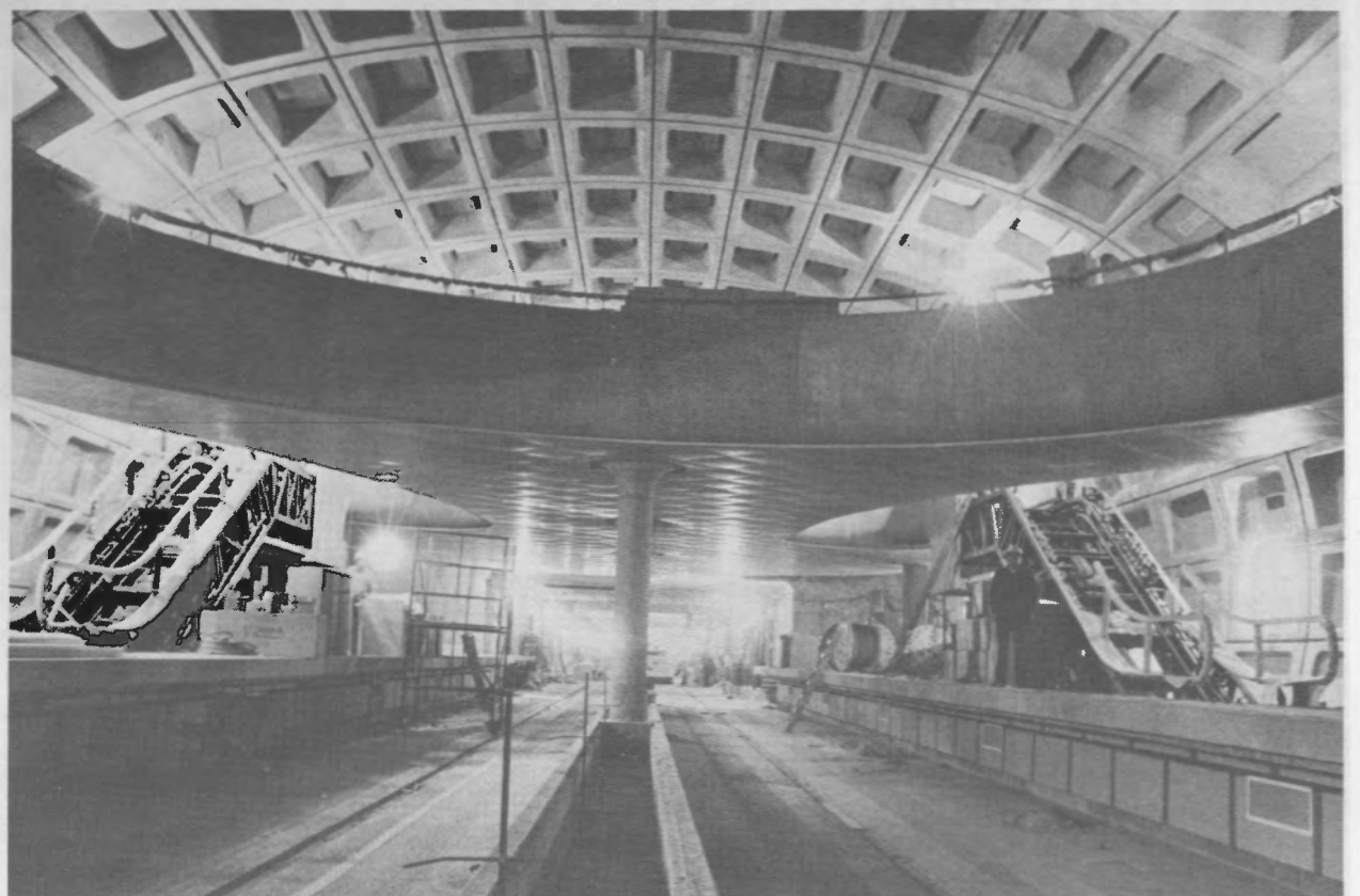
NEARING COMPLETION —Finish work continues on the Judiciary Square station. This side platform facility is among six stations to be opened in 1975. Passengers will pass through fare collection gates on the mezzanine (center) and descend to the train platforms on escalators seen under construction on either side of the mezzanine.
