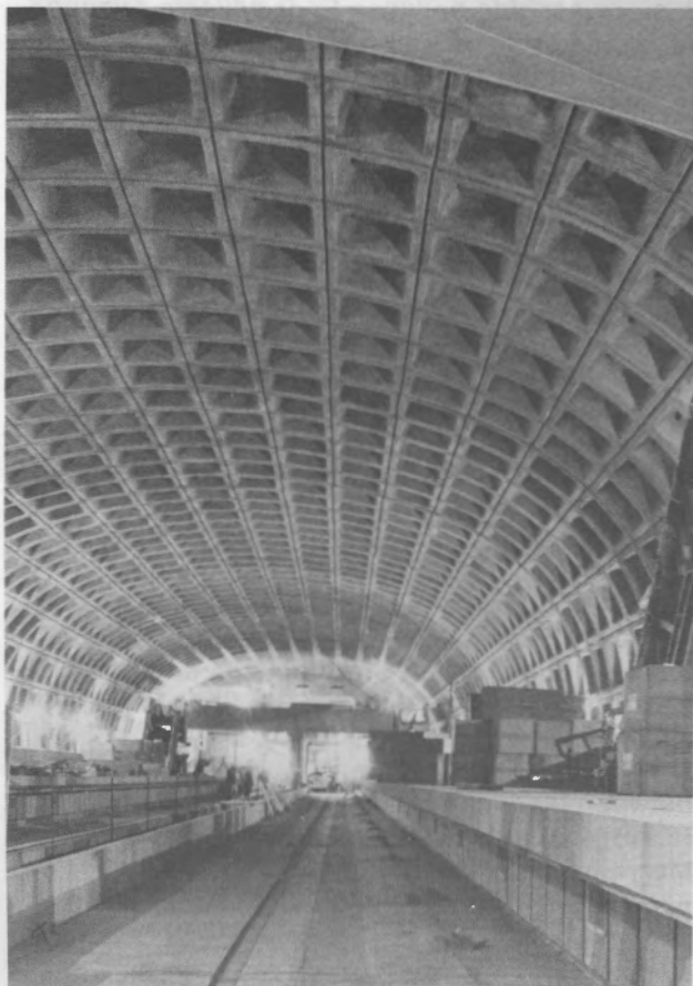
FLOATING SLABS —The concrete Metar trackbed (foreground) is mounted on vibration absorbent pads. Sound absorbent panels beneath the platform ledge at right will further reduce the sound of trains inside the stations. Continuously welded rail will eliminate the clackety-clack on the railroad track.
