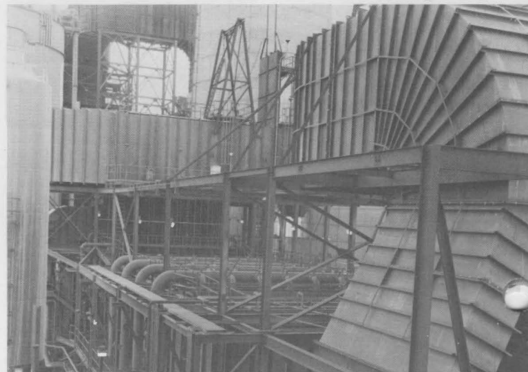
VIEW FROM THE TOP: A view across the top of the Weir scrubber shows the inlet flue gas duct (right) and the four headers (center) through which the slurry is pumped to the scrubbing section.
